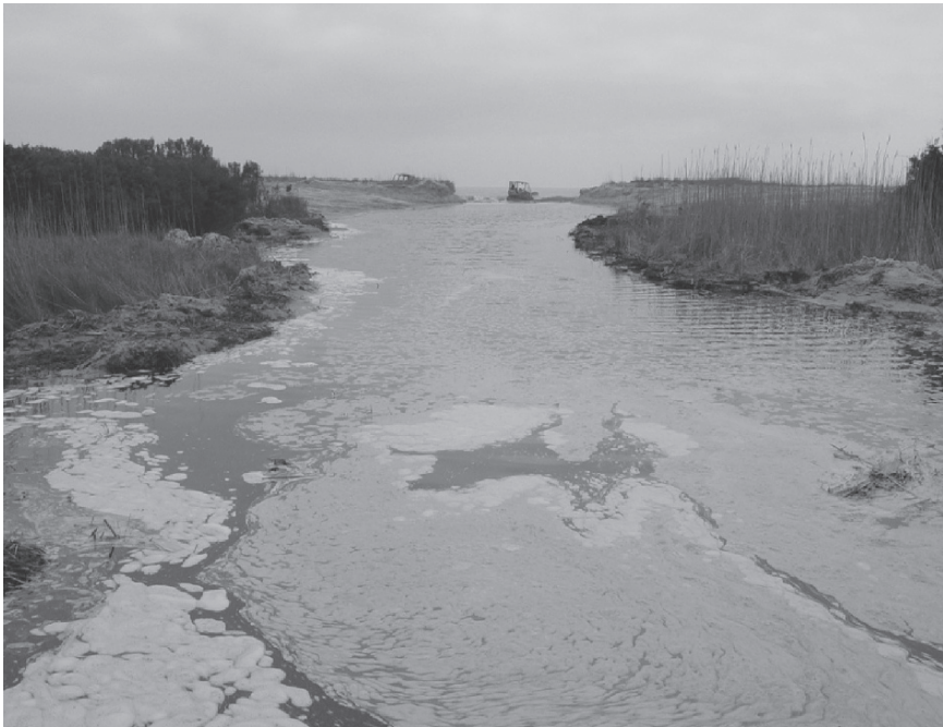
Fig. 4.3 The initial reexcavation of a channel from Sandpiper Pond through the barrier beach and extending into the ocean in April 2005. Stands of P. australis surround either side of the inlet and the excavator is located just in front of the ocean
